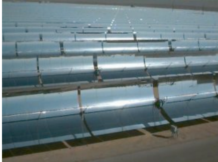
Figure 1: Rows of Thermal Collectors.
